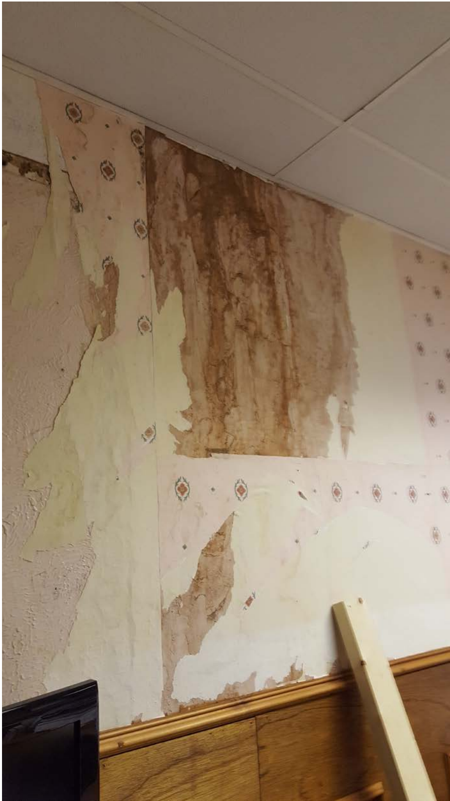
General condition of the walls in the dining area and evidence of a water leak.
