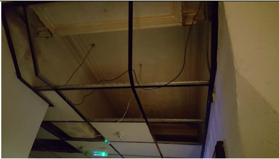
Ceiling tiles in the main reception hall, unsightly condition rather than dangerous.
